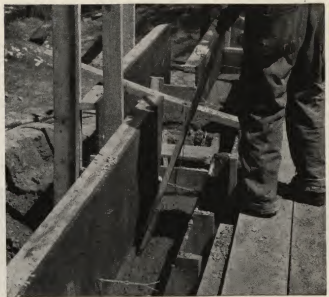
Thorough spading of concrete along form faces helps assure smooth, watertight concrete walls.
